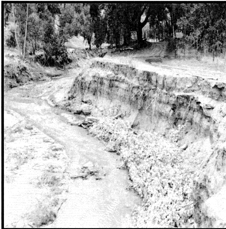
Figure 12. Site of potential road failure due to bank erosion, Canyon del Muerto. 96-0025WPF
