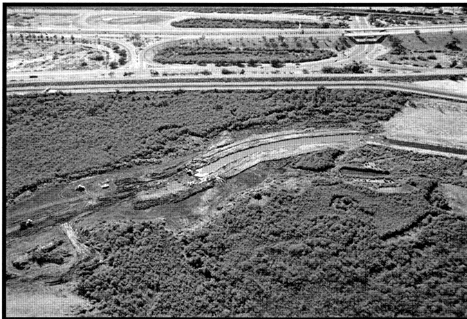
Figure 29. Overview of invasive vegetation removal and restoration activities along the Lower Colorado River at the Yuma East Wetlands Restoration Project. 04-124WPF
