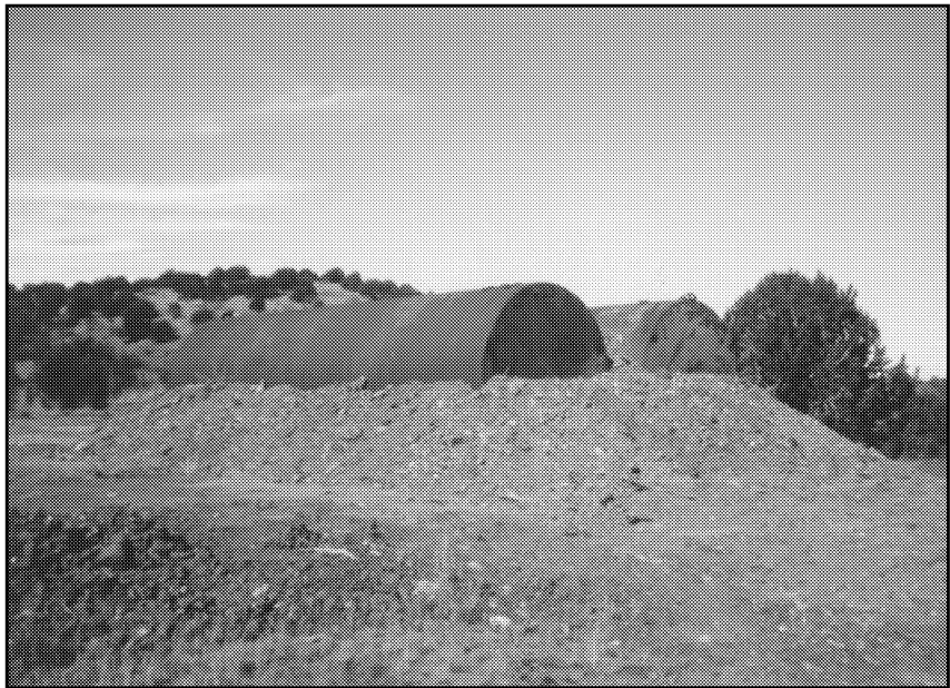
Figure 16. Two 20,000-gallon storage tanks to provide water replacement facilities upland. 98-047WPF
