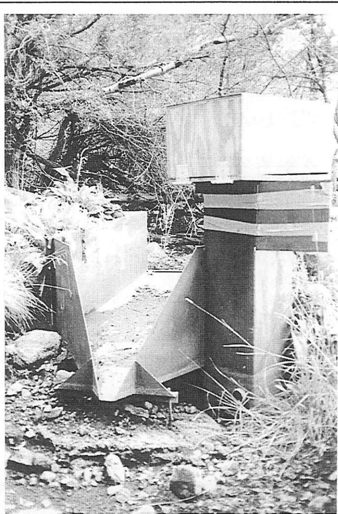
Figure 10. Flume installed to measure stream flow at Hart Prairie. 95-005WPF.
